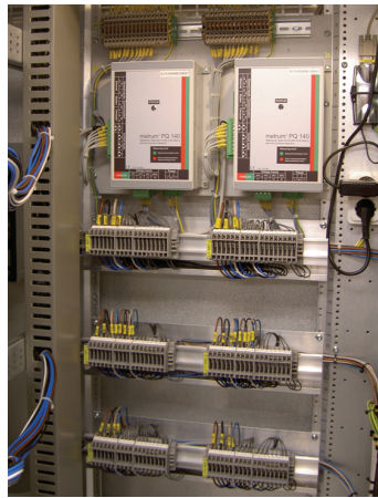
Fig. 8. PQ measurement devices installed in a substation (Source: Metrum)
